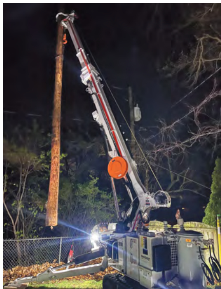
Local 245 members working to repair storm damage and restore service to their area.
