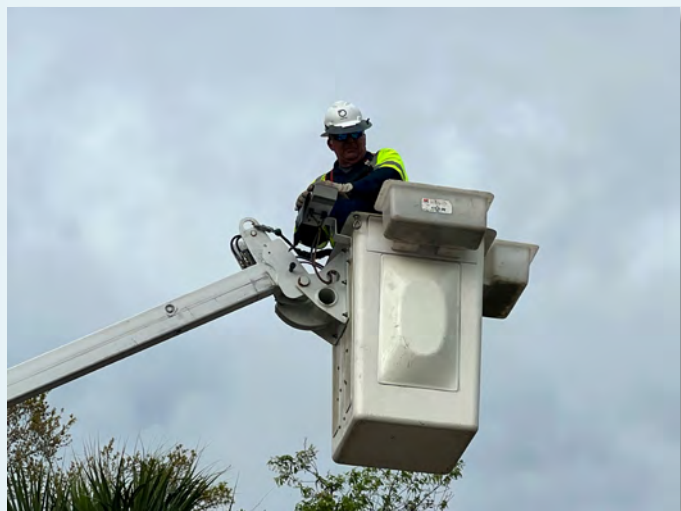
TELECOMMUNICATIONS Josh Saladino | Tampa, Fla., Local 824
