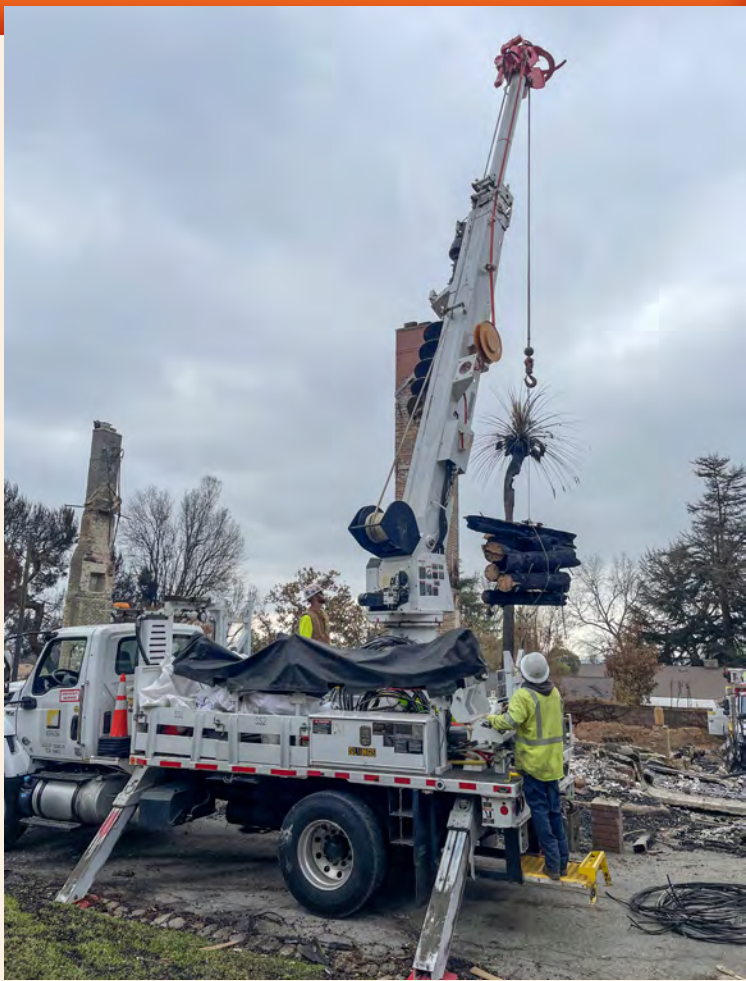
Local 47 line crews worked 16-hour days, seven days a week for up to eight weeks, rebuilding the distribution network, all too often for homes that were little more than concrete slabs and a chimney stack.
