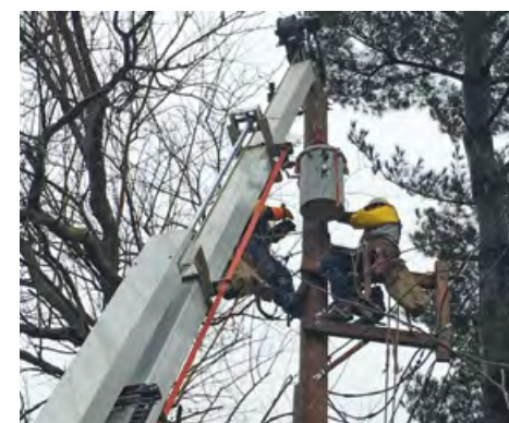
Local 245 members working on storm restoration on Toledo Edison/First Energy property in Ohio.
