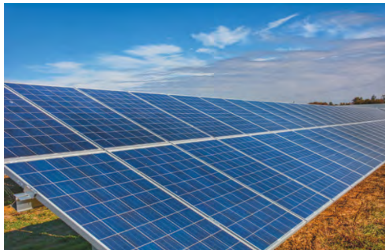
The IBEW recently saved the day for a utility-scale solar project in Ohio, just one of the scores of such projects being planned for rural communities throughout the state.
