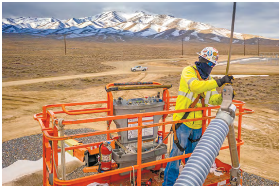
Local 1245 Lineman Dennis Scroggins works on the nation's largest DC-coupled combined solar and battery storage system, located in Battle Mountain, NV.
