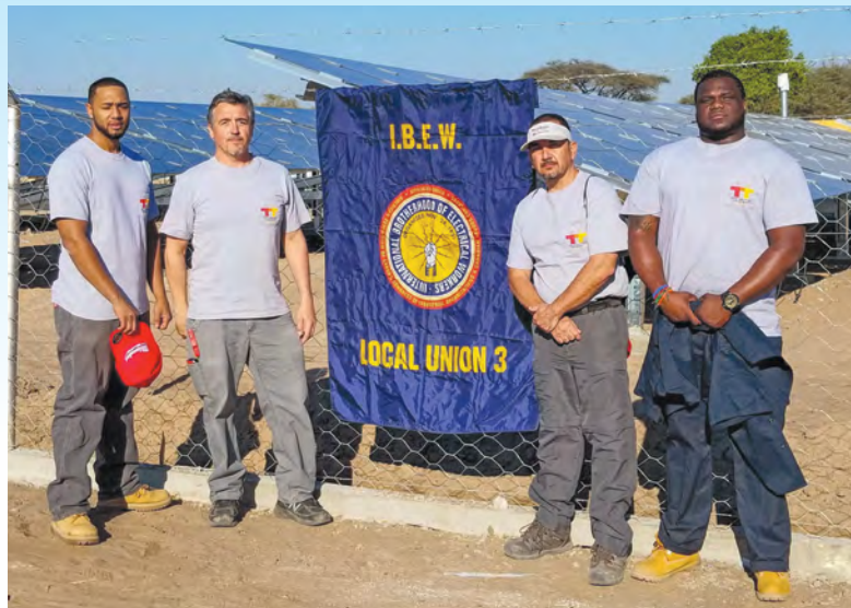
From left, Local 3 members Everest Campbell, Lou Alvarez, Alex "Archie" Alcantara and William Bonaparte show their IBEW pride in front of the solar grid they helped install at Chiulo Hospital in Angola in southwest Africa.
