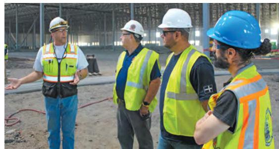
General foreman Dean Speelman (left) conducts tour of Home Depot project for IBEW Local 24 Bus. Mgr. Pete Demchuk, ETU National Apprenticeship Officer Mark Burgess and ETU outstanding apprentice Jack Todaro.
