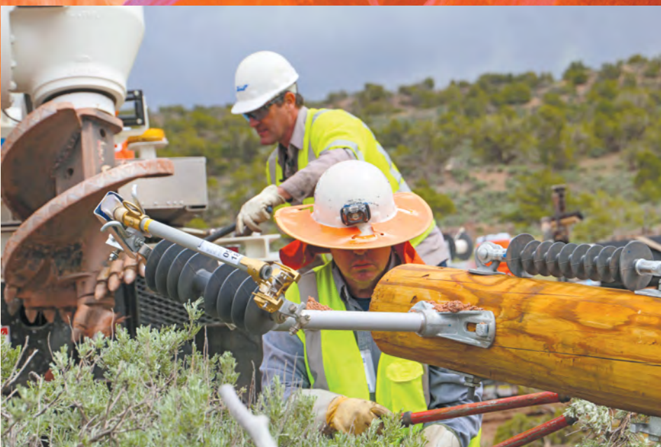
Phoenix Local 266 members Jayme Baranek and Mario Lizarraga, foreground, prepare to install a pole. They were among 30 members of their local at the Salt River Project who took part in Light Up Navajo.
