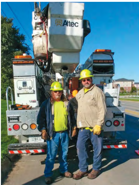
Local 55 members Dennis Gamble (left) and Robert Yeager, who work with the City of Ames, Iowa, Municipal Utility, get ready to install a new 900-amp G.O.A.B. air-break switch for circuit control.
