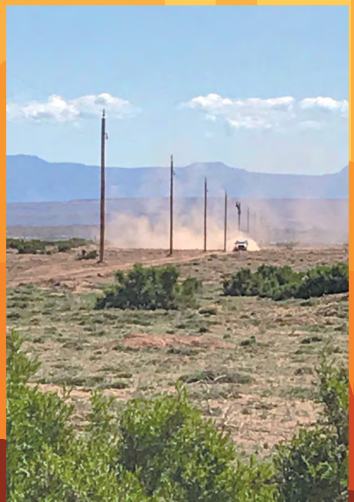
Worcester, Mass., Local 486 member Brian Foley's view of some of the estimated 1,000 poles that visiting utility crews working with NTUA electricians erected over six weeks in April and May across 50 miles of Navajo Nation terrain.
