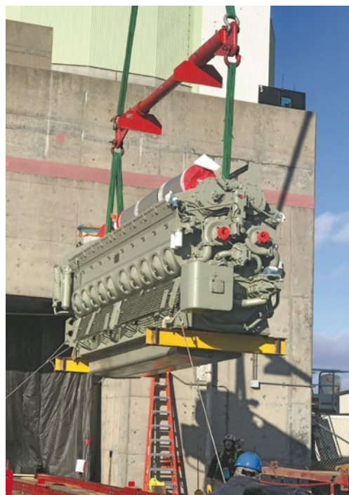
The nearly 25-ton engine block was craned into the nuclear station during the job, which required hundreds of electrical connections and even more teamwork.
