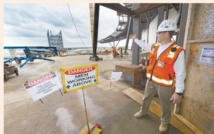
Federal OSHA is responsible for safety and health enforcement at construction sites, like this one at National Harbor outside Washington, D.C. Since this Department of Labor photo was taken in 2016 during a safety event attended by DOL officials, the number of OSHA inspectors has hit a historic low, reducing oversight and consequences for rule-breaking employers.
