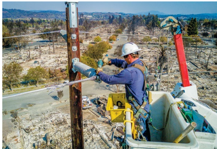
PG&E crews repair power lines damaged by the 2017 Tubbs Fire near Santa Rosa, Calif.
