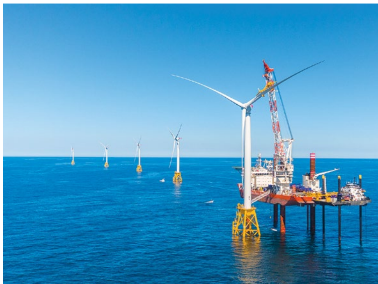
The Block Island Wind Farm under construction in early 2016. Icebreaker Wind, a similar project planned for Lake Erie, would be the first freshwater wind farm in North America and could add jobs for IBEW members.
