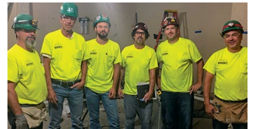
Local 38 Einheit Electric crew working at Q Arena transformation project: Don Atkins (left), Bob Wolf, Derek Barr, Dave Ball, steward Nick Heidenhoffer and foreman Mark Hanna.
