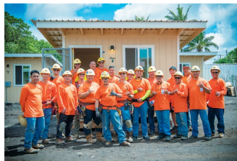
Members of Honolulu Local 1186 were among nearly 200 volunteers who helped build 20 tiny homes for residents displaced by the erupting Kilauea volcano earlier this year.
