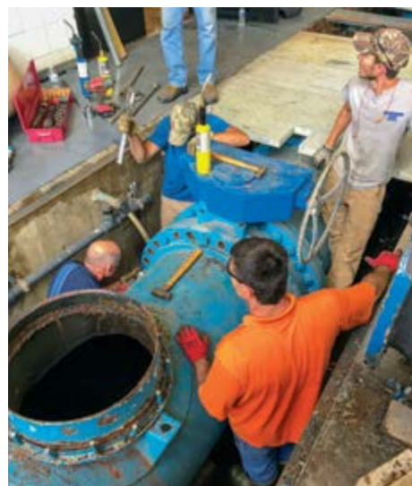
Local 702 members Dennis Toth (far left, crouching) and Dylann Vaughn (left, wearing blue shirt), along with several other members, worked 48 consecutive hours repairing a water main exiting the water treatment plant at Rend Lake Conservancy District.
