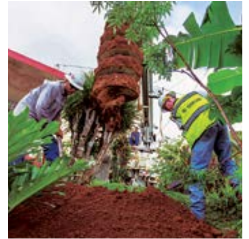
Local 1245 members Levi Schoennauer, Paul Duncan and Brent Sambel setting a pole in Puerto Rico. Credit: Sacramento Municipal Utility District.
