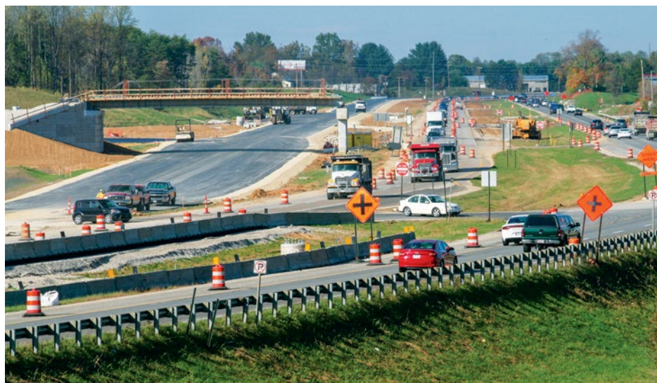
Work continues on the I-69 extension near Bloomington, Ind., in 2017. Changes to Indiana's common wage laws led by former governor and current Vice President Mike Pence have harmed workers on public works projects and their families.
