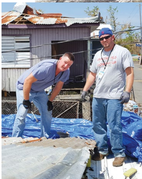
Volunteers repairing the HVAC system on the roof of San Juan Municipal hospital (top); Local 3 members Kevin and Patrick Glennon repairing the roof of an elderly couple (left), and a celebration the night before the first group returned home.
