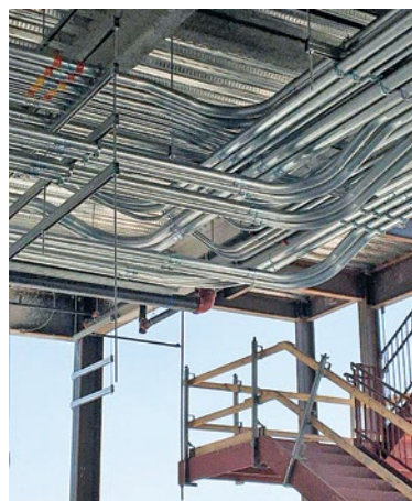
A view of conduit racks and runs installed by Local 570 members on fourth floor of Medical Center Towers project.
