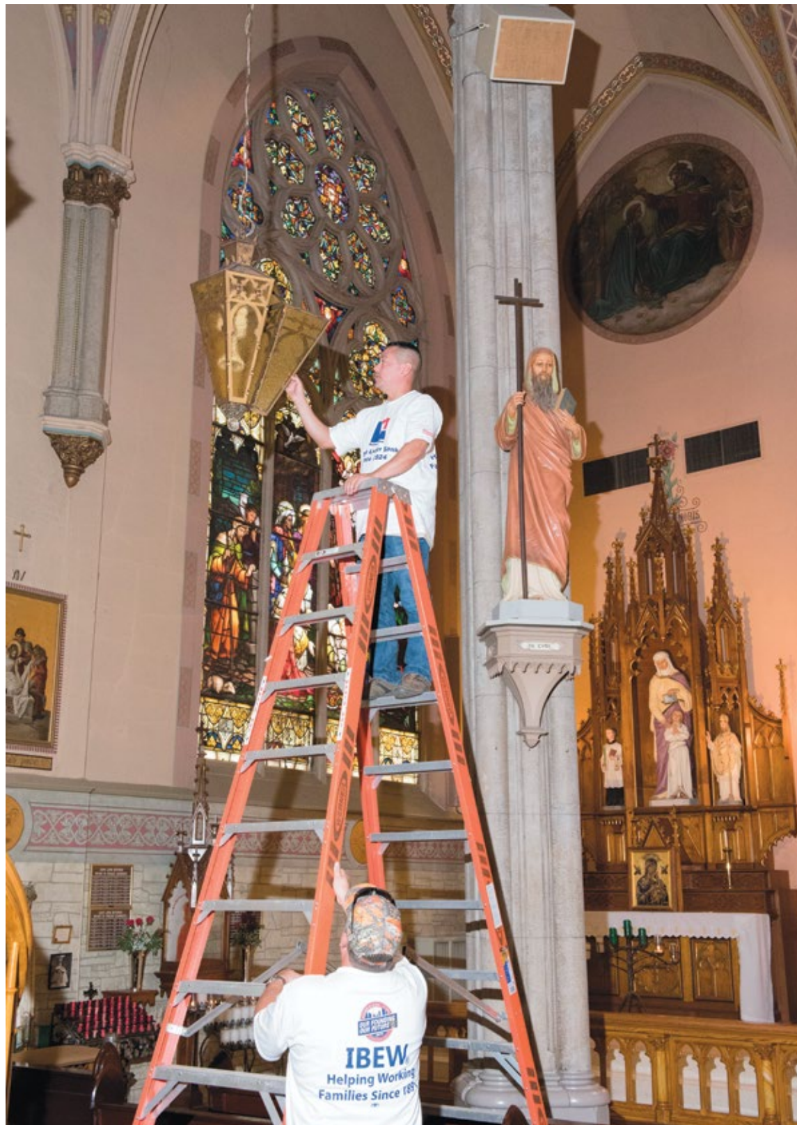
IBEW volunteers fanned out across the city to more than two dozen sites, but the largest was upgrading the community center, school and sanctuary of Our Lady of the Holy Cross church.
