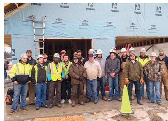
Local 557 members working with Leddy Electric volunteered to help build the Roberts Park Pavilion in Saginaw, MI.
