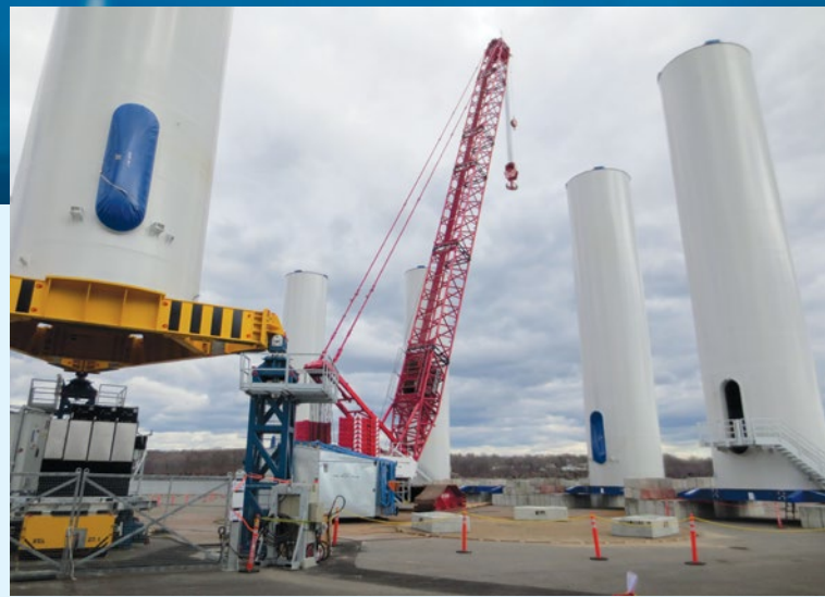
The bottom section of platforms that will support windmills at Block Island Wind Farm at the Port of Providence. They will be moved to the permanent site this summer. Above is an artist's rendering of the wind farm when it is finished. Graphic provided by Deepwater Wind.
