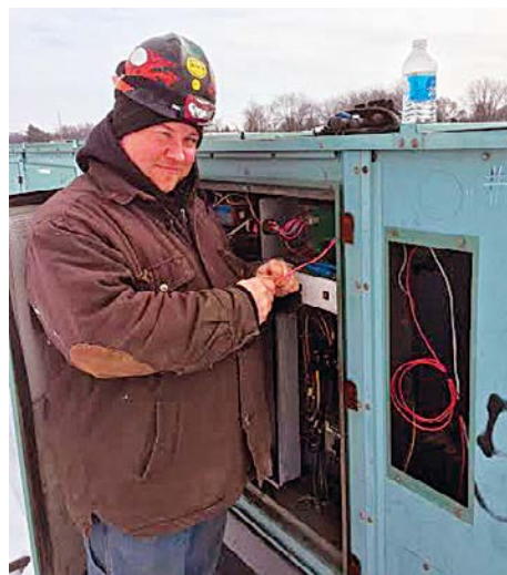
L.U. 557 journeyman wireman Mike Wesolek works on a fire alarm at the Kmart building in Saginaw.
