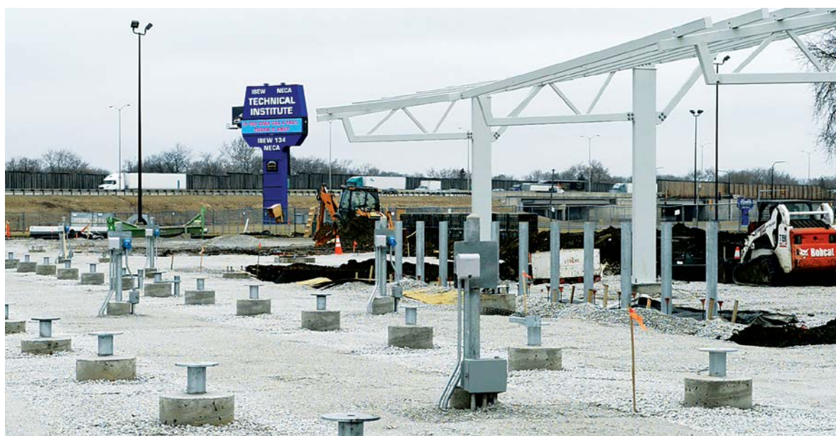
Chicago Local 134's training center will soon boast state-of-the-art training in solar, wind, building automation and smart metering technologies.
