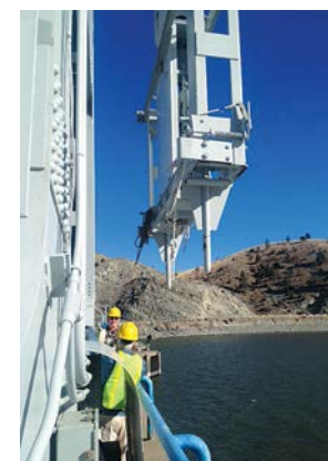
Local 1759 Bros. Jeff Lord and Jack Hatcher lower a lifting device down to a river outlet gate at Canyon Ferry Dam.
