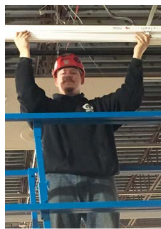
Local 557 member Nick Iles installs new lights for remodeling project at Kmart building in Saginaw, MI.
