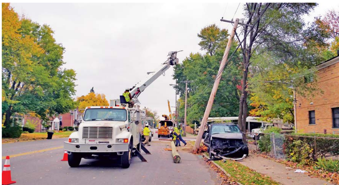
Members of Detroit Local 17 are modernizing the city's electrical infrastructure—building by building.
