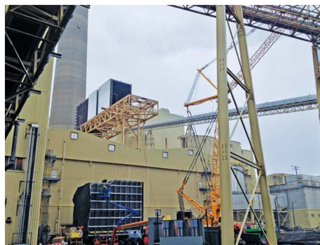
Local 388 members are working on Weston 3 power plant's ReACT emission control project.
