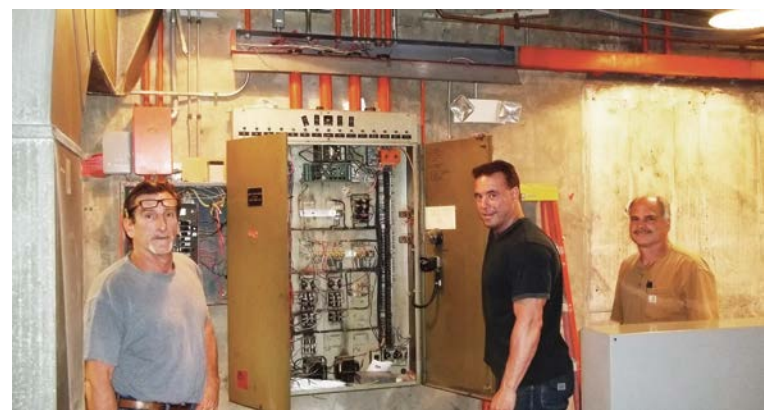
Local 38 members Kevin O'Toole (left), Chris Chilia and Jim Zito, from Zenith Systems, work on the power and temperature control for Local 38's newly renovated HVAC system.
