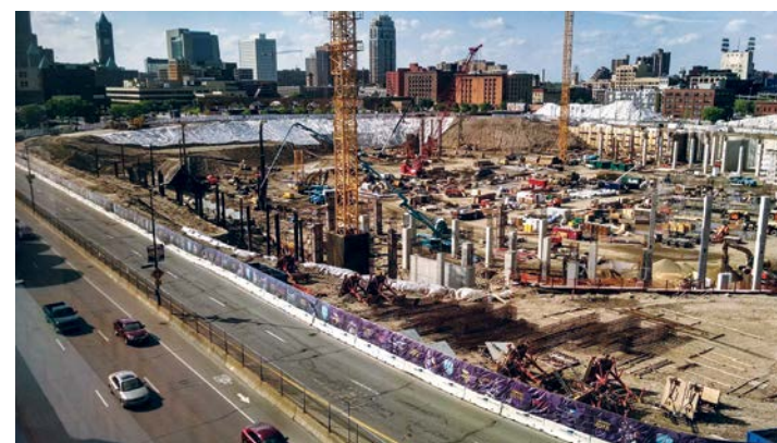
With the help of IBEW Local 292 members, the Vikings People's Stadium is on schedule for completion in 2016.
