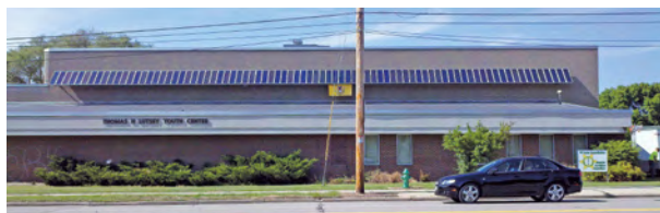
IBEW Local 158 volunteers installed solar panels at Green Bay Boys & Girls Club.
