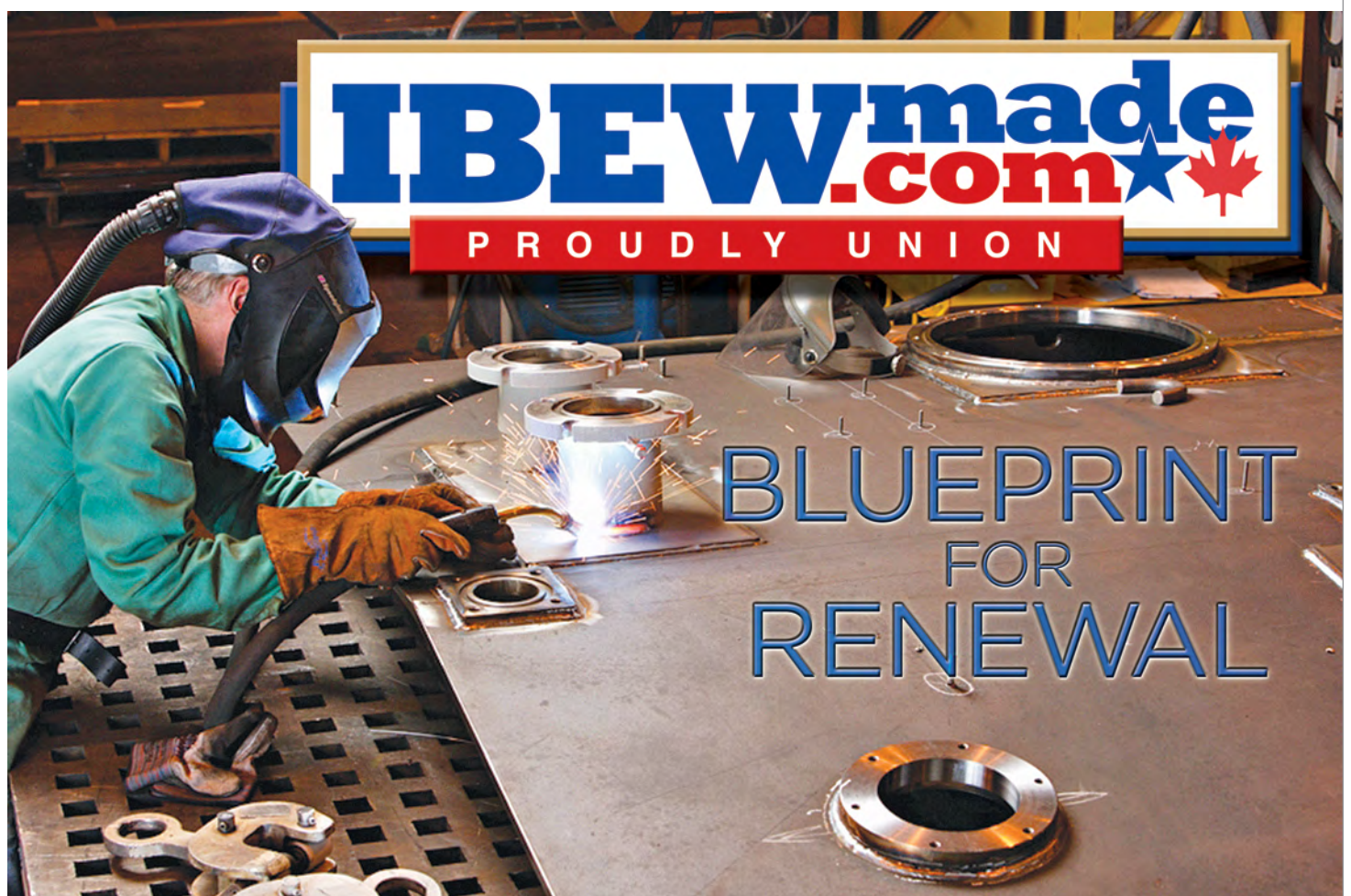
The IBEW and SPX Transformer Solutions in Waukesha, Wis., are working together to grow union manufacturing.
