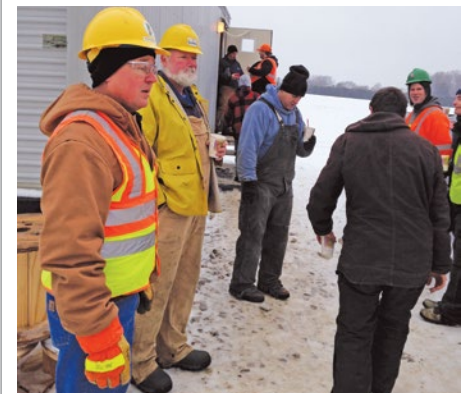
Local 300 Asst. Bus. Mgr. Tim Watkins (left) and Peck Solar General Foreman Vince Bent (second from left) thank IBEW members for giving their all on a cold Saturday.
