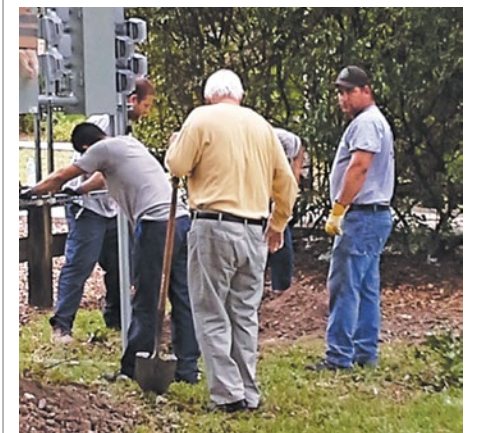
Members of Locals 222 and 349 install underground electrical service to supply power for Christmas decorations and a tree lighting ceremony at library.
