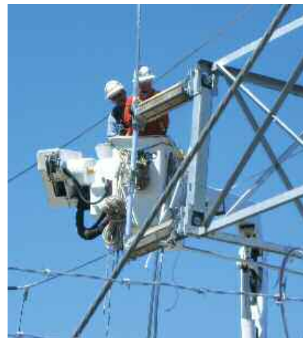
IBEW linemen Scott Downer and Dillian Irvin at work on a Local 659 project with ILB Inc. at Lone Pine substation in Medford, OR.
