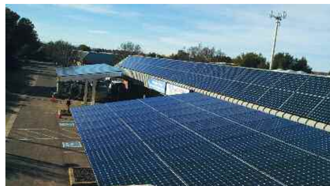
IBEW Local 340 Training Center's PV/Solar Parking Canopy installed by Cal Valley Solar, Schetter Electric and Sac Valley Electric.
