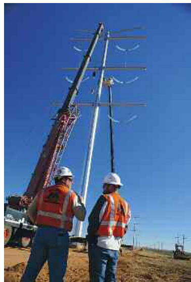
IBEW Local 898 Gen. Foreman Rodney Garcia (left) and Michels Corp. project manager supervise erection of one of 333 steel monopoles.
