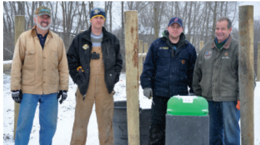
Lansing Local 665 apprentices helped install an automatic horse watering system at a therapeutic riding center.
