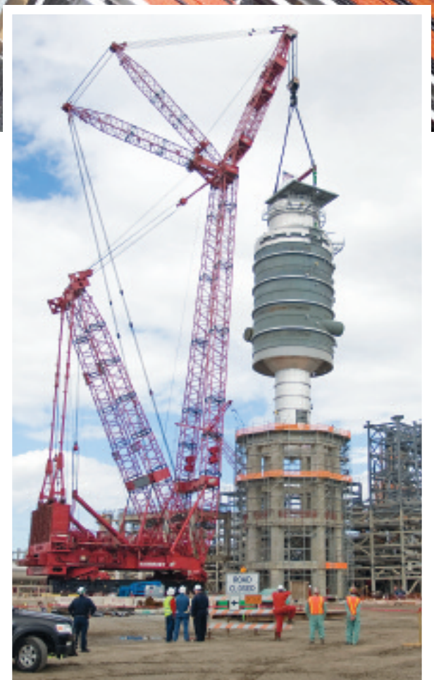
Gary and Hammond, Ind., Local 697 members and hundreds of travelers are working on a massive new BP refinery to process crude oil from Canada.
