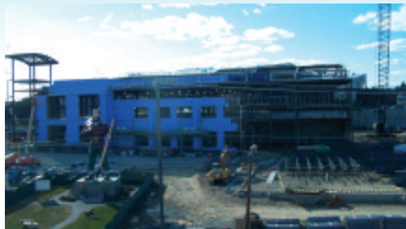
Construction is under way at the new convention center in Bangor, Maine, employing a number of IBEW Local 1253 members.
