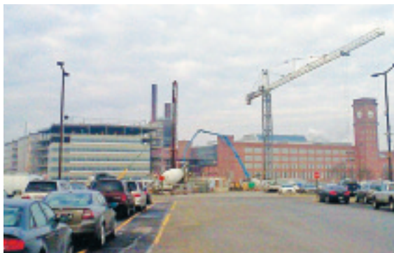
Goodyear Tire & Rubber Co. construction site, where IBEW Local 306 members and fellow trade unionists are working.
