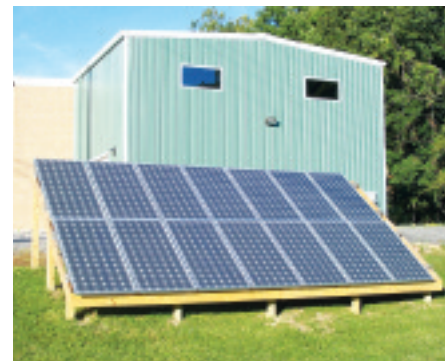
Local 596 JATC training facility includes solar panels installed for hands-on training.
