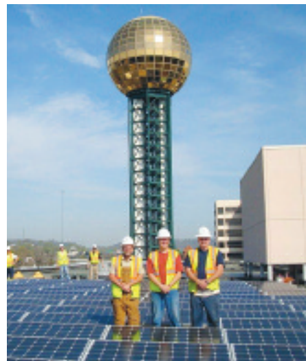
Local 760 Bros. Scott Whaley (foreman), Jack Badon (steward) and Gary Mykenson on solar installation project at Knoxville, TN, Convention Center.
