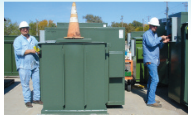
Local 1523 journeyman meter man Jeff Harris (left) and first-year apprentice meter man Tad Woodard at work on the job. Not pictured is Amy Poynter, second-year apprentice meter man.
