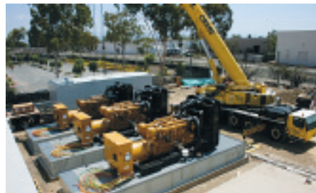
IBEW Local 441 electricians worked with Stout & Burg Electric Inc. on the big Latisys Data Center project in Irvine, CA.
