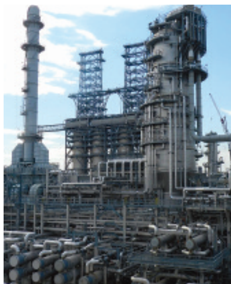
Local 649 wiremen, joined by IBEW traveling members, worked on the Coker Unit project at Conoco Phillips Refinery.
