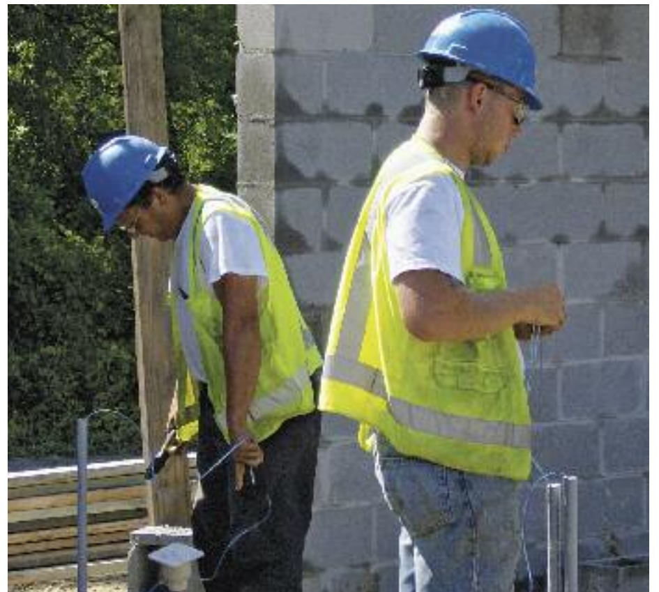
Frank Visconti, left, a construction electrician, and construction wireman Jimmy Martin work on a project in Jacksonville, N.C. for Blackwater Electric.
