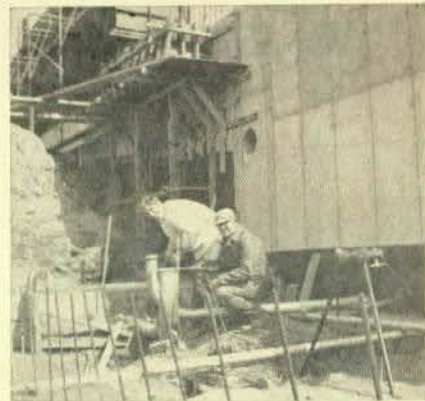
Left to right, are Bob Adams and Steve Fainer, working on the transformer-pad job at a new church in New Haven.
