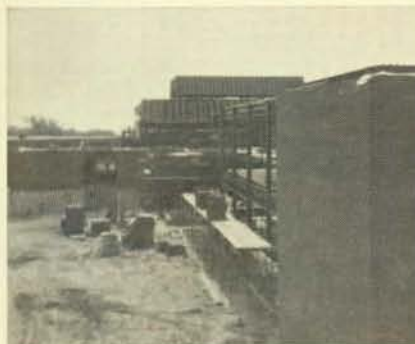
This is a view of the George Street Complex which will house the largest arts and music center in the Crawford County area.
