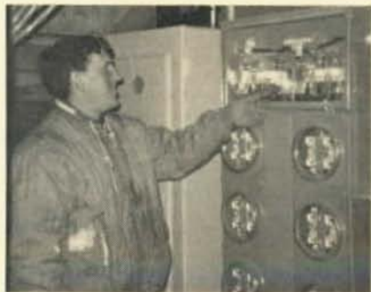
Douglas Bumforo, also employed by the Motor Shop Electrical Construction Company, checks a part of the meter panel on the Brown Brothers' Apartment Complex job in Battle Creek.
