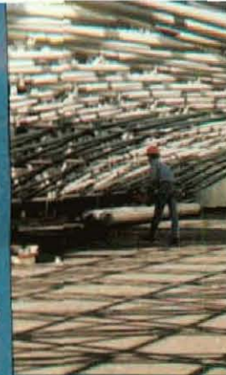
Most of the canopy is built on the ground. Working under it are (from left) General Foreman Lloyd Beadle, Journeymen Wiremen Steve Baggs and Tom Lowler, and apprentice Laura Willis.
