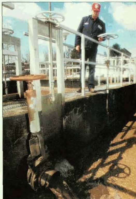
Local 300 member Sam Gates checks the valves at the Enosburg Falls Wastewater Treatment Plant.
