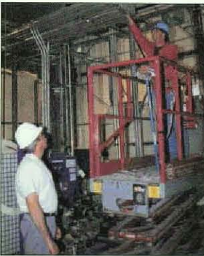
12 Electrical Superintendent Ron Gabrick (left) watches as Louis Poirer makes an adjustment at the Auburn Recycling Facility, an innovative project for Local 567, Portland, Maine.
