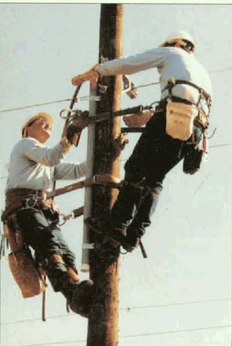
Journeyman Lineman for Kansas Power and Light and Local 304 member Scott Hildebrandt (left) and a co-worker up on a pole.
