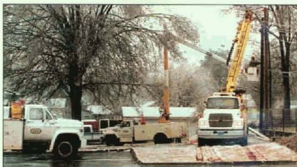
2 Local 558, Sheffield, Alabama, utility crews working to bring electric power to residents hard hit by the ice storm.
