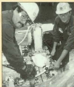
Local 1733, Fredericton, NB, members Kevin Desaulnier and Gary McLaughlin remove the turning gear assembly of the 350-megawatt turbine generator at Caleson Cove Unit #2 during an annual outage in 1993.
