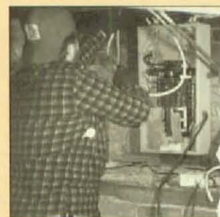
Local 481, Indianapolis, IN, Bro. John Bates Jr., along with other local union members, helped to rewire the home of an area family as a community service.
