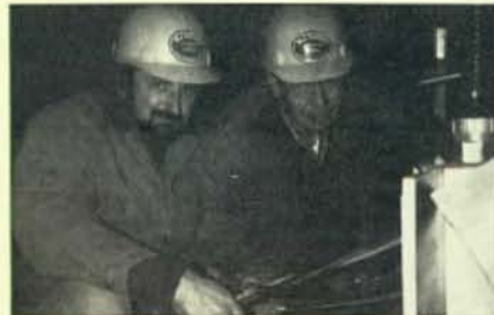
Brothers Richard McInerney, Local 494, Milwaukee, Wis., and Sam Dalgrehn of Local 276 are shown on motor termination.
