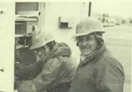
Journeyman Joe Quarantillo and foreman Joe Loterio working on a traffic signal controller for Buffalo, N.Y.
