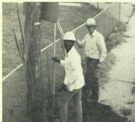
Ed Holms, lineman and past vice president, and Robert Jones, trainee, are putting another stick in the ground on Lafayette Boulevard.
