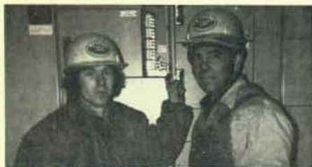
Working for M. J. Electric on the Louisiana Pacific job are Brothers John Kuss, Local 347, Des Moines, Ia., left, and Stephen Ronchak, Local 276, Superior, Wis.
