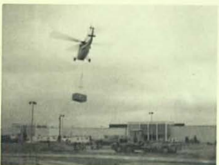
A helicopter taking one of many air-handling units to the roof of the shopping center.
