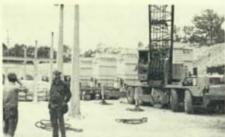
Members of Local 846, Chattanooga, Tenn., are working at the Falling Water Substation for the Chattanooga Electric Power Board. Here the riggers are setting transformers.
