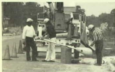
Shown is a complete crew of Local 980, Norfolk, Va. They are Linwood Askew, auger operator, with Bill Colbertson, groundman, and John Garris, lineman, setting lights where the old Hudgins Farm used to be in Virginia Beach.
