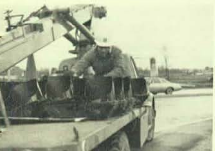
Apprentice Wes Stoddard getting signal lights ready to be hung. Wes works for Ferguson Electric in Buffalo, with Ken Bowers as foreman.
