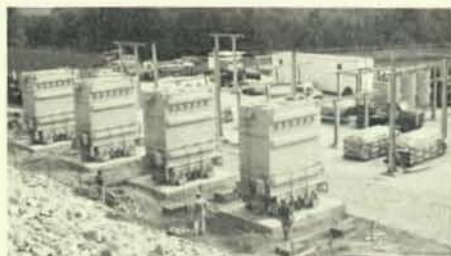
The Falling Water Substation.
