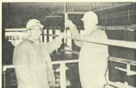
Brothers Charlie Cooper and Walt Wilson installing wiremold lighting track at Sears.
