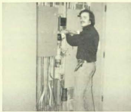
Apprentice Chuck Matson files in computer relays at Exchange Building.
