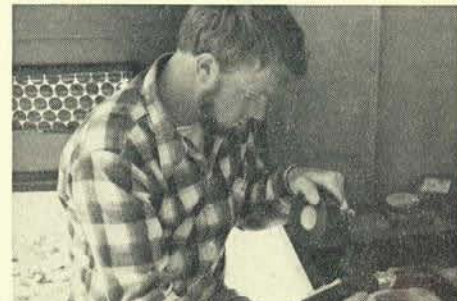
Brother Bob Fritz of Local 400, Asbury Park, N.J., wrapping high voltage splices.
