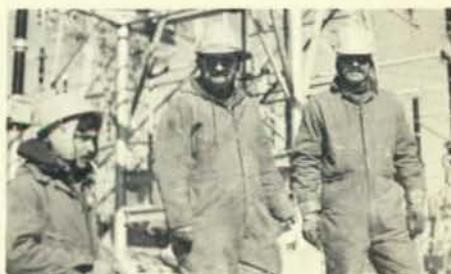
On the County Electric job at Pleasant Valley Substation, left to right, are Charles Douglas, Joe Hilyard, and Bill Oliver.
