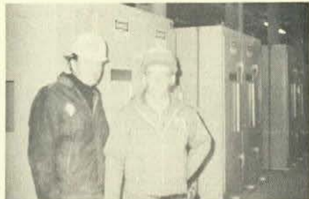
Matt Miller, general foreman, left, and Bernie Gnefkow are shown in the switchgear room at Sears.
