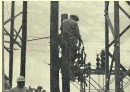
John Middleton and Roger Perry working at the Summerville Substation.
