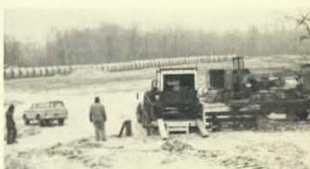
The T. D. Bross yard at Wappingers Falls, N.Y., high-line job. When this photo was taken they were just getting set up and receiving the wire.
