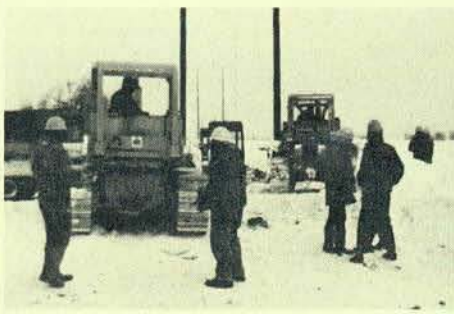
Melvin Garrett's framing crew at Bradley and Williams's job in Arcade, N. Y.
