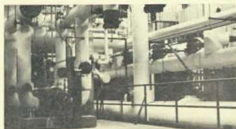
Hot water circulating pumps, heat exchangers, and chilled water lines are part of the equipment making up the heart of CSC's mechanical area.
