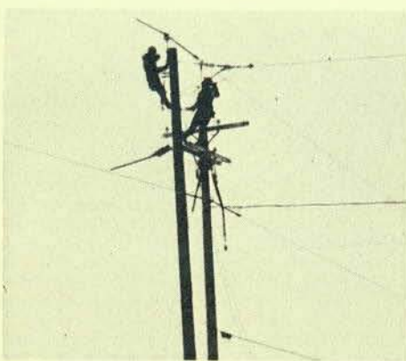
Tony Kota, journeyman, and George Warner, apprentice, revamping 2,400 to 19,900 on job at Fillmore.
