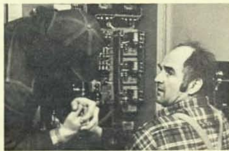
Brothers Steve Bersing, left, and Bob Feuhling connect an emergency generator transfer switch.
