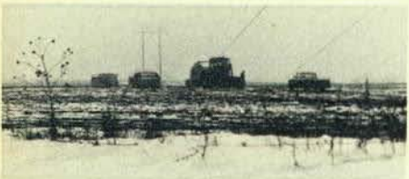
These photos show members of Local 55, Des Moines, Ia., pulling wire on reconductoring job between Boonville and Ashawa substations for Hoak Construction Company.
