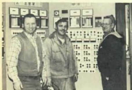
Shown at the Waukegan Sewage Treatment Plant in front of the master monitoring panel, wired by Local 150, Waukegan, Ill., men. Left to right are Brothers Tom Otterson, Dick Bouma, and Burt Nielson.
