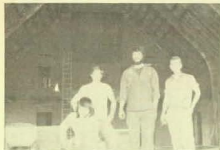
Here Brothers Norm Kipker, Jim Reynolds, Al Smith, and Vern Sutherland, left to right, show that they do go to church, every day. This site happens to be the new Zion Lutheran Church being built here in Lima, Ohio, by Local 32 members.
