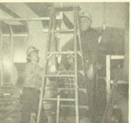
Mike Orban, on ladder, Ed Kepczynski, left, and Tom Schmalz, rear, install the 12-inch cope trays for the 500 mcm. This picture was taken in the utility tunnel to the new four-story office building at C. R. Braun and Company.
