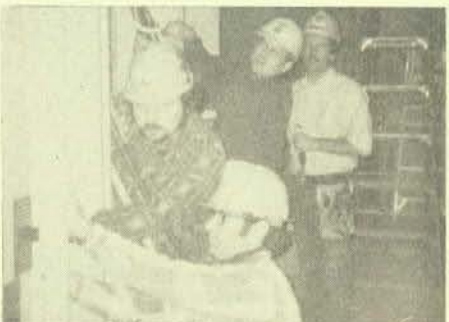
Members of Local 262, Plainfield, N.J., working for F. L. Baumeister Electrical Company, prepare to pull nine more "legs" of 500 mcm at C. R. Braun and Company, Murray Hill, N.J. Front to rear are Pat O'Donnell, John Gorel, Ken Derr, and Paul Greaves.
