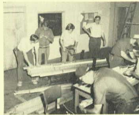
These Brothers contributed some 60 hours of labor installing lighting and small power equipment at the Noble Sheltered Workshop in Indianapolis; left to right, Barry Payne, Jack McCullough, Steve Alsmeyer, Bob Sterling, Bill Kijovsky, Richard Curfman, and Matt Rasnick.
