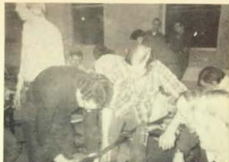
Local 181, Utica, N.Y. recently held a splicing school at Utica Free Academy. Here journeymen are shown working on 15-KV splice.
