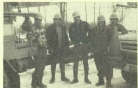
Local 300, Montpelier, Vt. members shown here on the job in Rutland, left to right, are Bunky Richards, Sid Disorda, Trapper Young, and Joe Frankiewicz.
