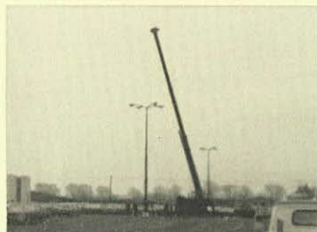
Local 773, Windsor, Ont. members are employed at new Chatham Place Mall. Here light standard is put in place.
