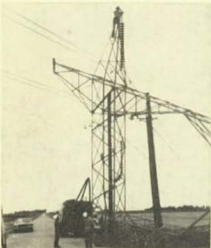
Tom Ganzer, Stan Horsfall, Louis Pederson, and Jim Thompson (in the air), Local 55, Des Moines, Ia., work on one of the downed towers.
