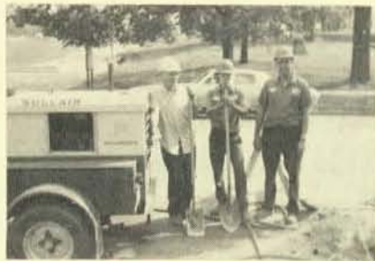
Left to right, foreman Homer Rhodes, Bob Labelle, and Seth Goodhue, Local 300, Montpelier, Vt., gas workers, are on the job in Burlington, Vt.
