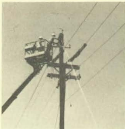
Jim Kinzel and Charlie Middleton catch off wire on a new deadend pole on a reconductoring job in Des Moines.
