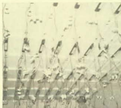
These are the dimming fluorescents in the new conference room; Dennis Ragen is shown in background.
