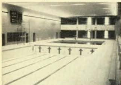
New swimming pool is lighted by 17,000 watts of mercury vapor lighting. Total of 7,000 fixtures in school installed by men of Local 229, York, Pa.
