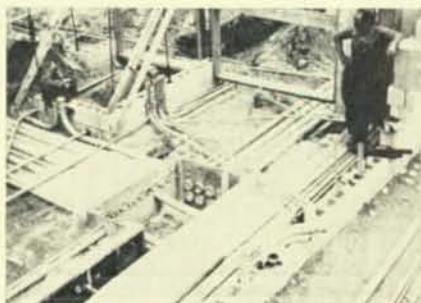
The mains and the sub-mains in the slab of the electric room.
