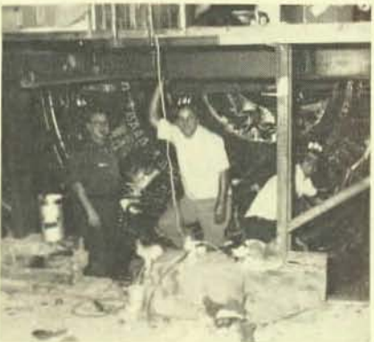
Brother Joe Gerald, "Wild Bill" Pulaski, and Joe Sanford complete work on generator of Unit 2, Zion Nuclear Station.
