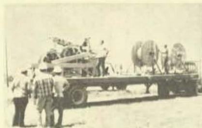
Local 55 members string wire under tension for the Hoak Construction Company in Des Moines.
