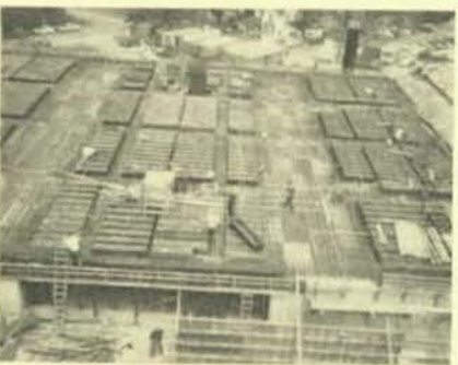
An early photo, showing the crew starting to pipe in one of the decks of the Learning Complex.
