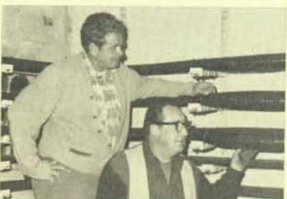
Splicer Ted Day, left, and assistant Larry Brennan inspect some of their splices on 11-KV sub-feeds.
