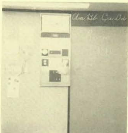
A typical nerve center, showing a school system clock, light switches, a thermostat, a public address speaker, a radio and TV receptacle, an FM broadcast jack, and a telephone for the interphone system.
