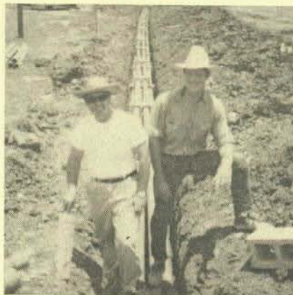
Left to right, G. A. Morgan and R. L. Wilkins demonstrate a new method of holding pipes in dikes by using cement blocks.
