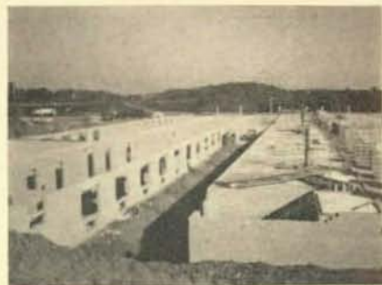
The first floor of the two-story, 134-unit motel, Shenandoah Inn, in the jurisdiction of Local 299, Cambridge, Ohio.
