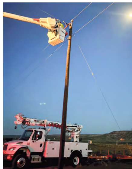
Local 483 members representing the IBEW at the Light Up Navajo project.
