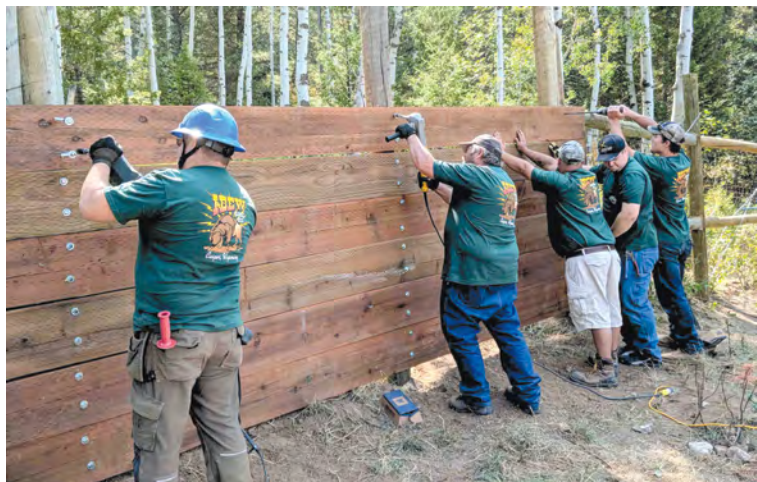
Volunteers from Casper, Wyo., Local 322 construct a custom elk jump at a state feeding ground, a project spearheaded by organizer Bruce Johnson, whose conservation efforts were honored this spring by the Union Sportsmen's Alliance.
