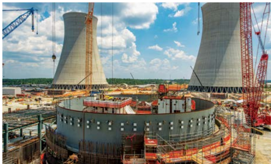
Out-of-work Canadian members could get the chance to work on construction of Plant Vogtle, a nuclear station under construction in Georgia, alongside members from Augusta, Ga., Local 1579.
