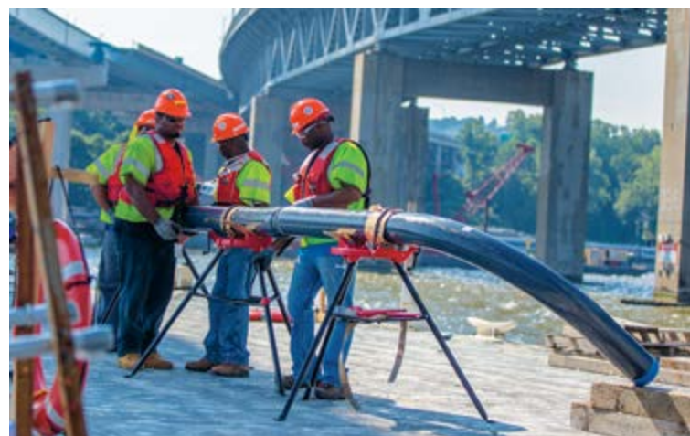
Members of New York Local 3 and New City, N.Y. Local 363 shared the electrical work. Here, workers assemble conduit on a temporary floating platform.
