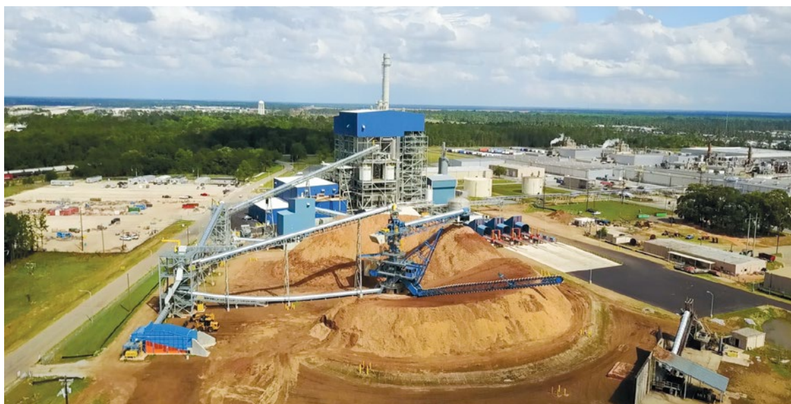
A 50-megawatt biomass facility owned by Constellation Energy under construction in Albany, Ga.
