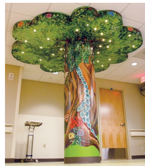
IBEW Local 375 members worked on construction of a decorative "tree" at Children's Oncology Suite at Lehigh Valley Health Network.
