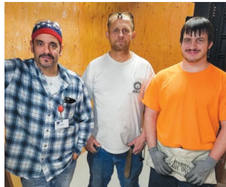
Local 673 members Tony Gambatese (left), Kevin Saunders and Nick Capuiso at Old Kaiser Building jobsite.
