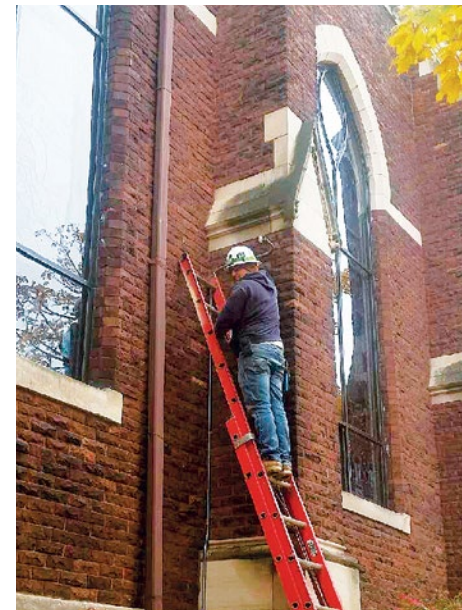
IBEW Local 557 member Rex Christian at work for Thiel Electric on lighting at St. Mary's Cathedral in Saginaw, MI.
