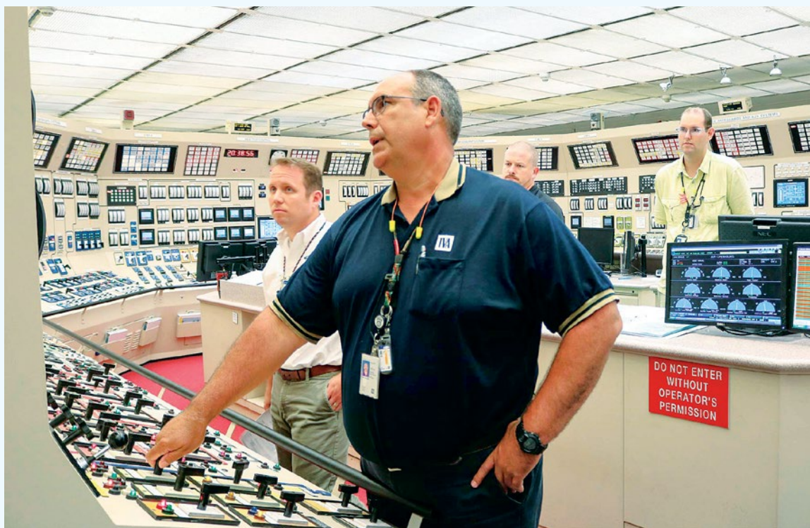
Reactor operator and Rockwood, Tenn., Local 1323 unit steward Bill Hahn mans the control room during Watt's Bar Unit 2's first moments producing energy.
