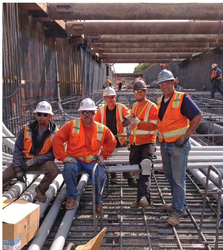
Members of San Jose, Calif., Local 332 are engaged in a four-year project extending Bay Area Rapid Transit service by 10 miles.
