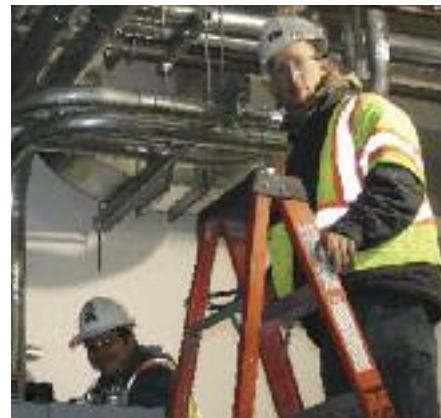
Local 82 members working at Wright Patterson Air Force Base for ESI Electrical Contractors include journeyman Lucas Bates (left) and apprentice Gabe Thomas.
