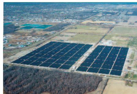
Sarnia, Ontario, Local 530 members, joined by travelers from five sister IBEW locals, completed the first phase of a huge solar farm with additional work scheduled for spring.
