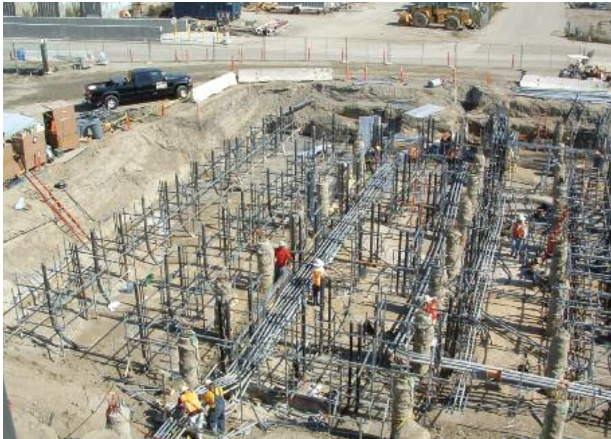
More than 150 Santa Ana, Calif., Local 441 members worked on Orange County’s new wastewater treatment plant, which converts wastewater into drinking water.
